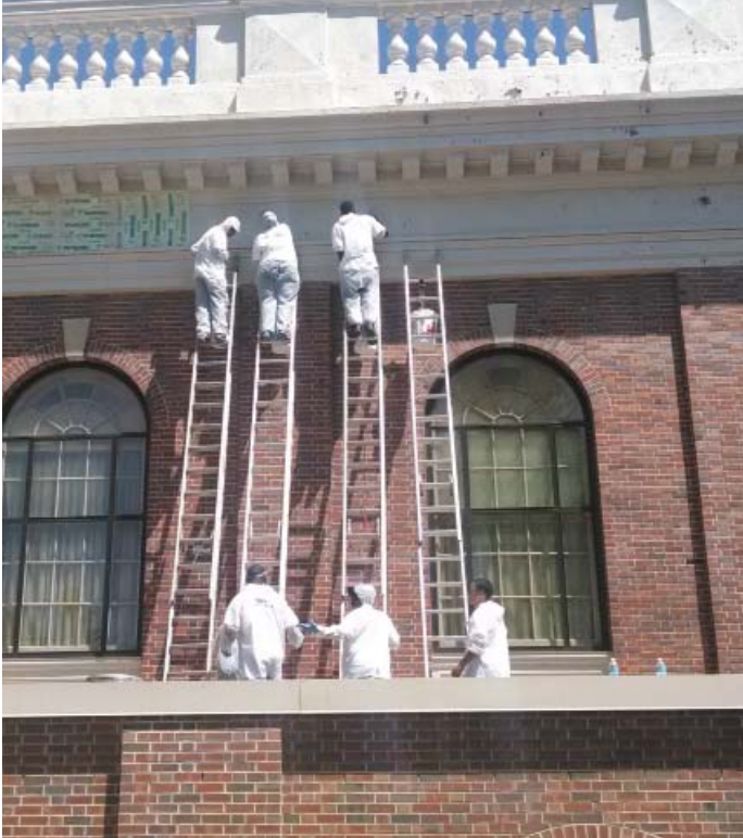
Above: On May 29, workers scaled ladders to strip and prime surfaces before a new coat of paint.
